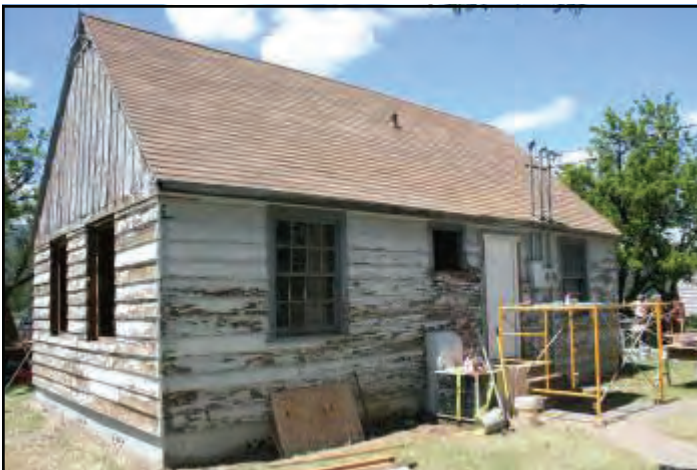
The administration building as it appeared before June 2010 restoration by National Smokejumper Association volunteers.
